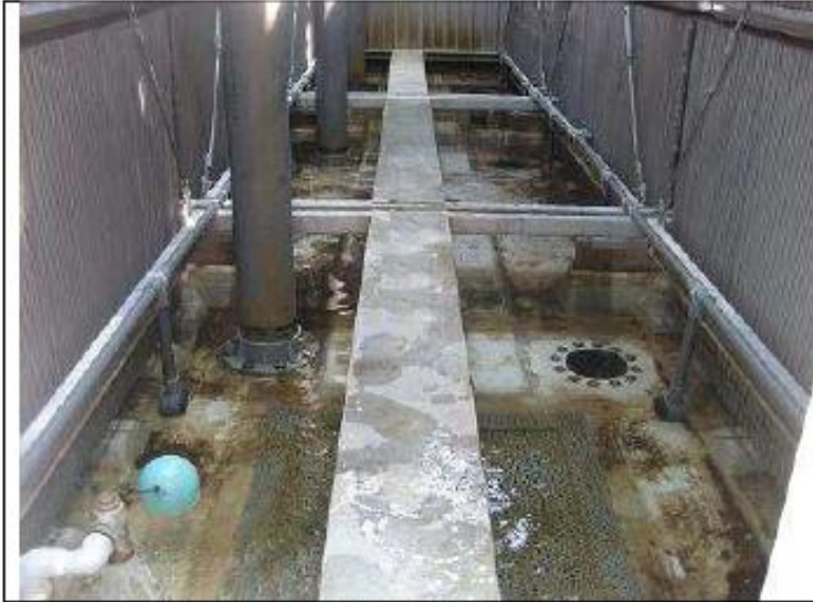
Figure A: Emitter Layout in Big Cooling Tower
