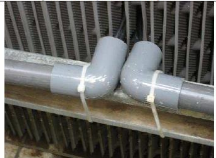
Figure D: Cable Penetration thru Fin of Cooling Tower
