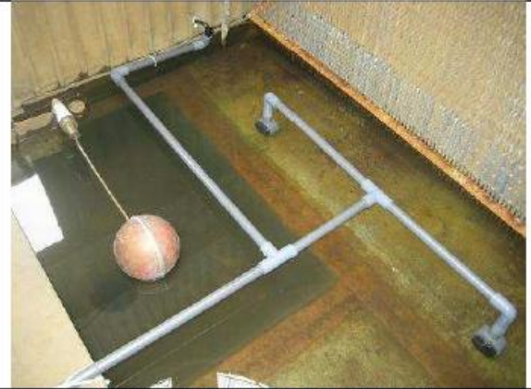
Figure B: Emitter Layout in Small Cooling Tower
