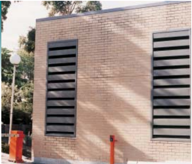
H-Line Louvres reducing plant-room break out noise
