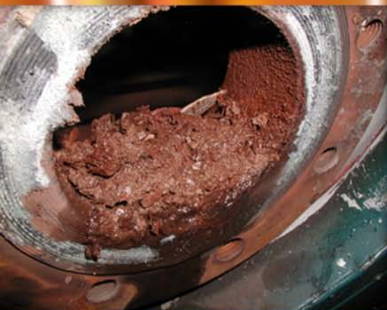
Descaled Scale Fragment from Fire Tube Boiler
